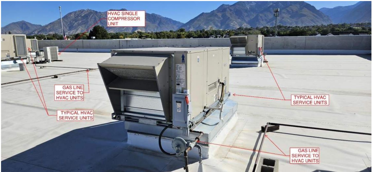
FIGURE 28 - MULTIPLE ROOFTOP HVAC UNITS
