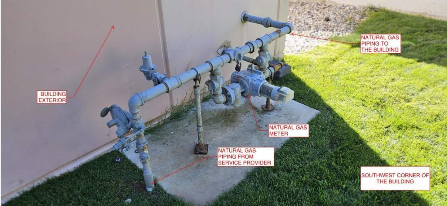
FIGURE 19 - NATURAL GAS SUPPLY METER
