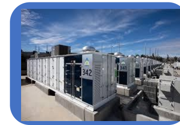
Other Technology: storage, grid management, etc.
