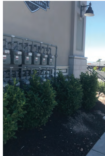
Figure 1105 - Wall-mounted equipment screened by landscaping
