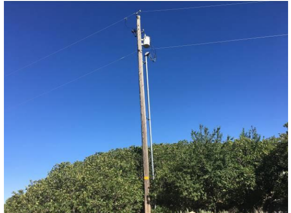
Photo #16 Pole-mounted transformer on the southeast side of the site.
