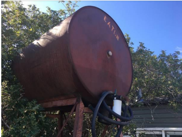
Photo #25 500-gallon diesel AST on the site.
