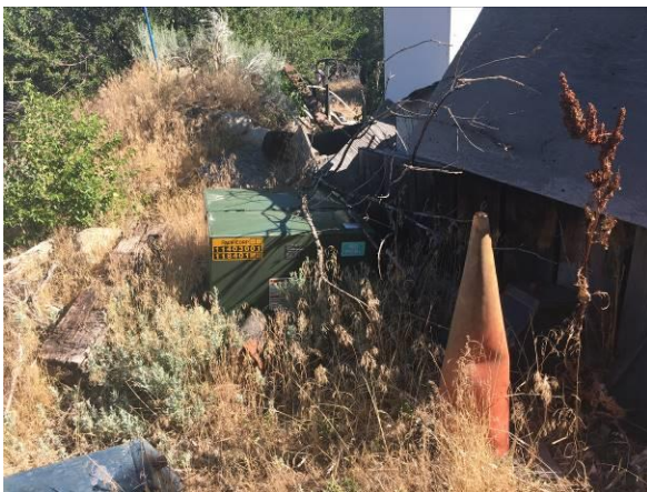
Photo #35 Pad-mounted transformer on the west side of the site.
