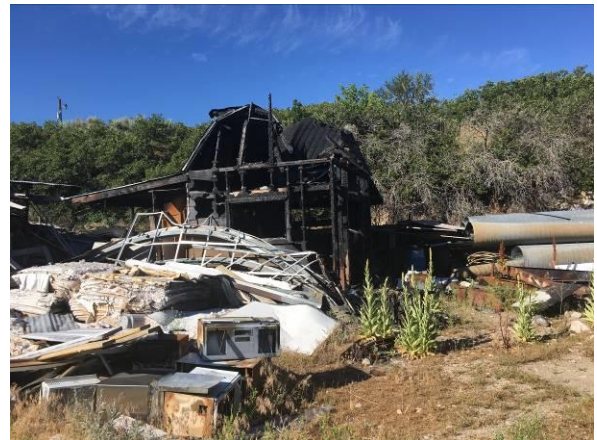
Photo #22 Structure that burned in a fire.
