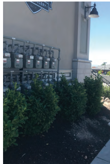
Figure 1105 - Wall-mounted equipment screened by landscaping
