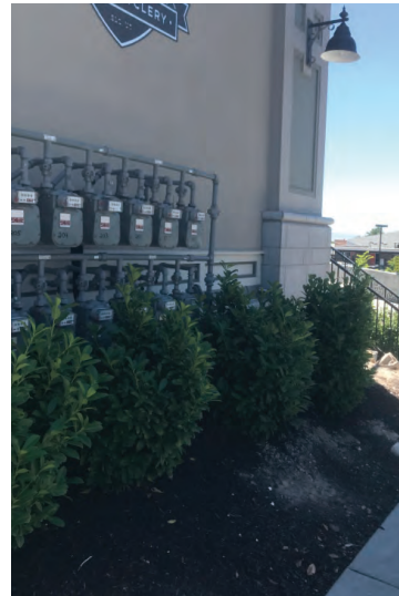
Figure 1105 - Wall-mounted equipment screened by landscaping
