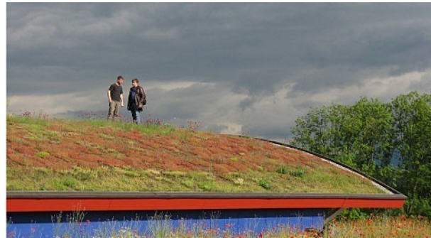
Green roofs are unique stormwater features which also provide a variety of diverse benefits to building systems as well as inhabitants and users.
